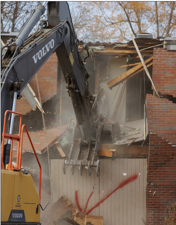
Demolition on the A Building of the Grove Apartments began Dec. 4, with work on the C Building and the B Building to follow. The demolition work is expected to be completed in the next few months.
