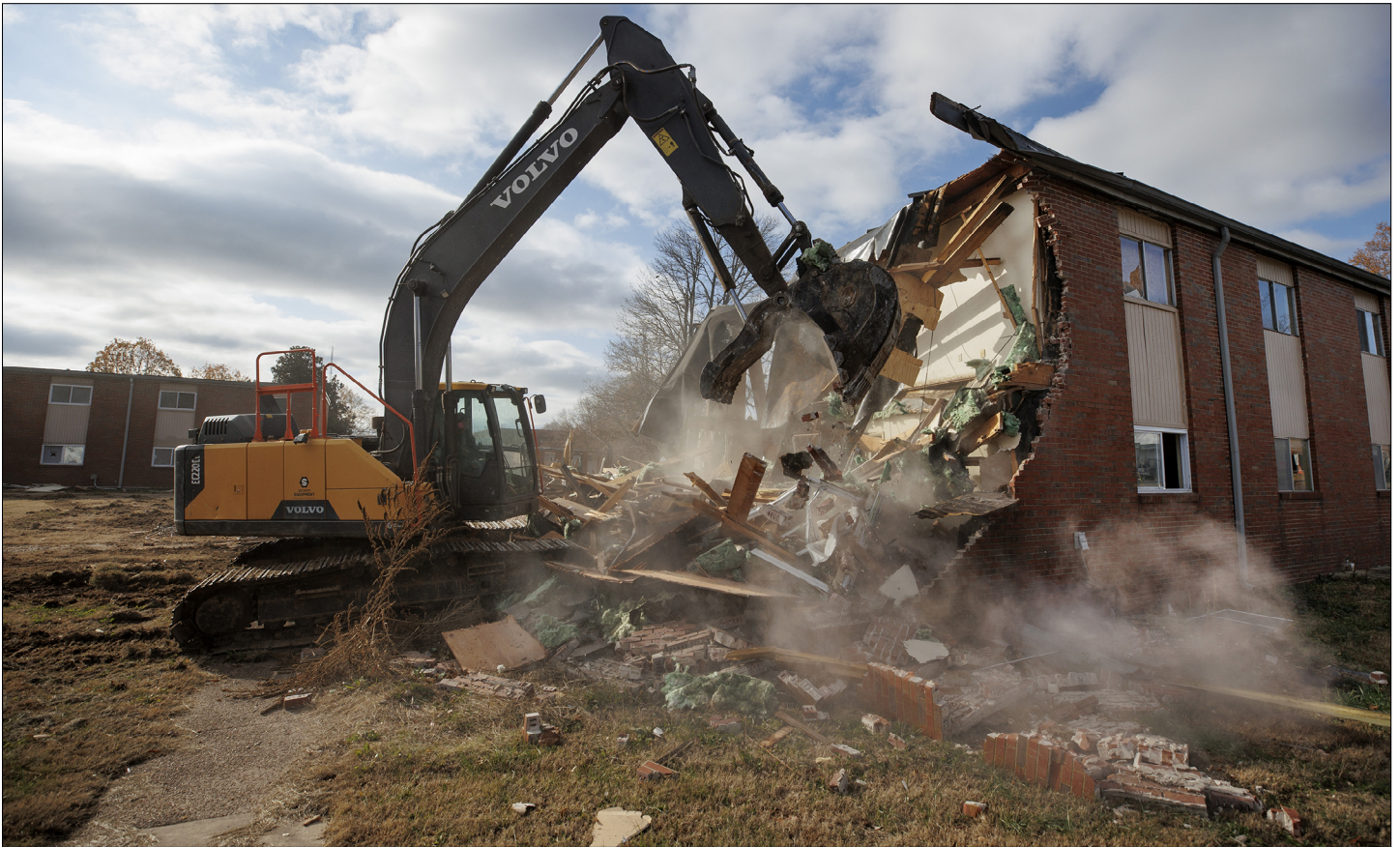
Demolition began Dec. 4 on the Grove Apartments, a residential complex that has stood for 58 years at UT Martin.
